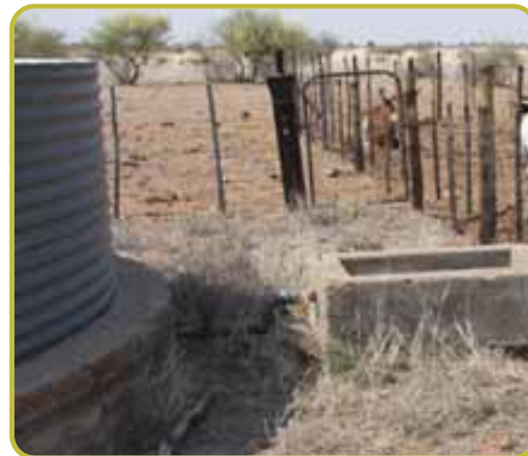
Photo 67: Troughs refill quickly if the diameter of the pipes and the distance between reservoir and trough is short. Also notice that the ball valve is not in the trough, but in a separate box in a fenced area so that animals cannot damage it.
