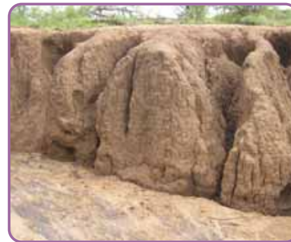
Photo 9 Gullies cut deep into the landscape.
